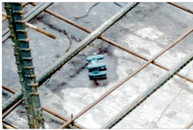
Figure 5 – Spacer that tumbled during a concreting operation
