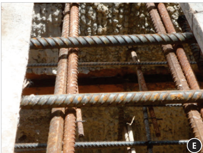
Detail of hydro swelling flexible tape already placed for next concreting procedure: reinforcement for next concreting phase is totally completed
