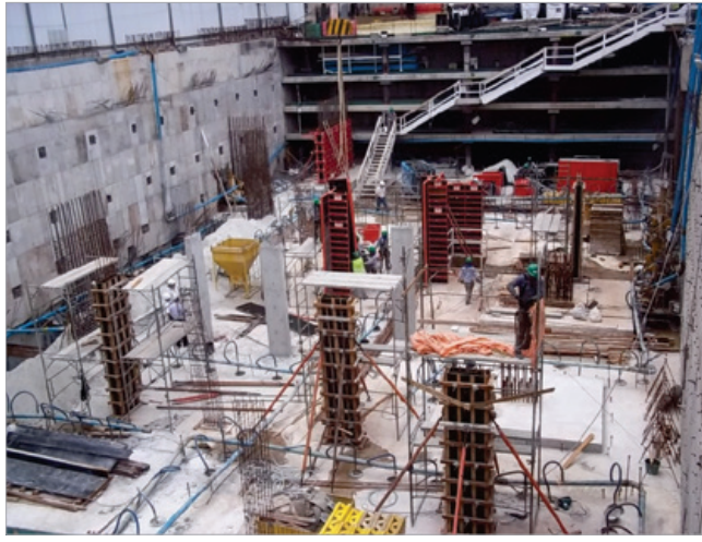
Figure 6 – Anti-flotation slab already finished and beginning of formwork erection of 2nd basement columns (some of them already concreted)
