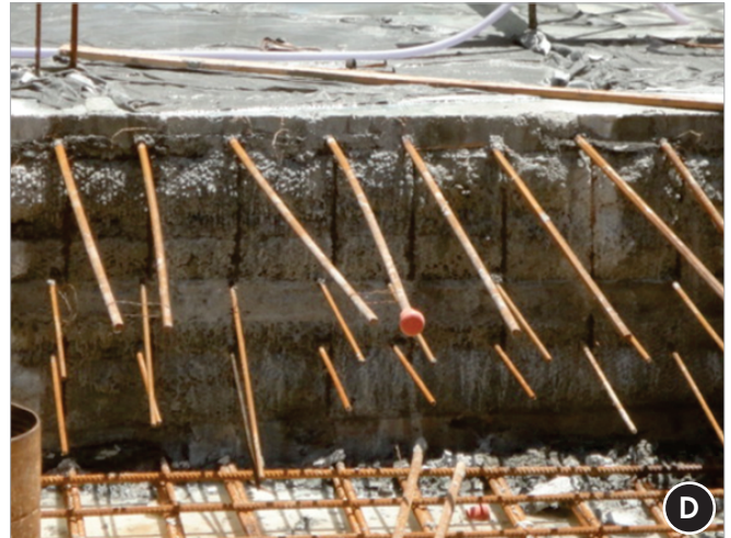
Detail of concreting joint before hydro swelling tape placing: vertical and rough surface, the next slab reinforcement not yet finished
