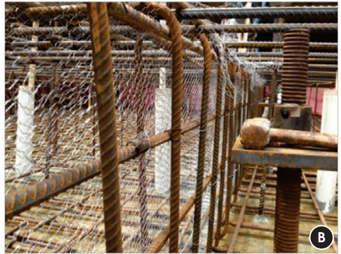
Detail of concreting joint with poultry wire mesh and external reinforcement support
