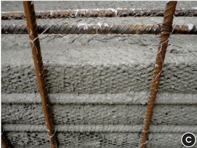
Detail of poultry wire mesh performance during concrete placing: minimal cement slurry leakage
