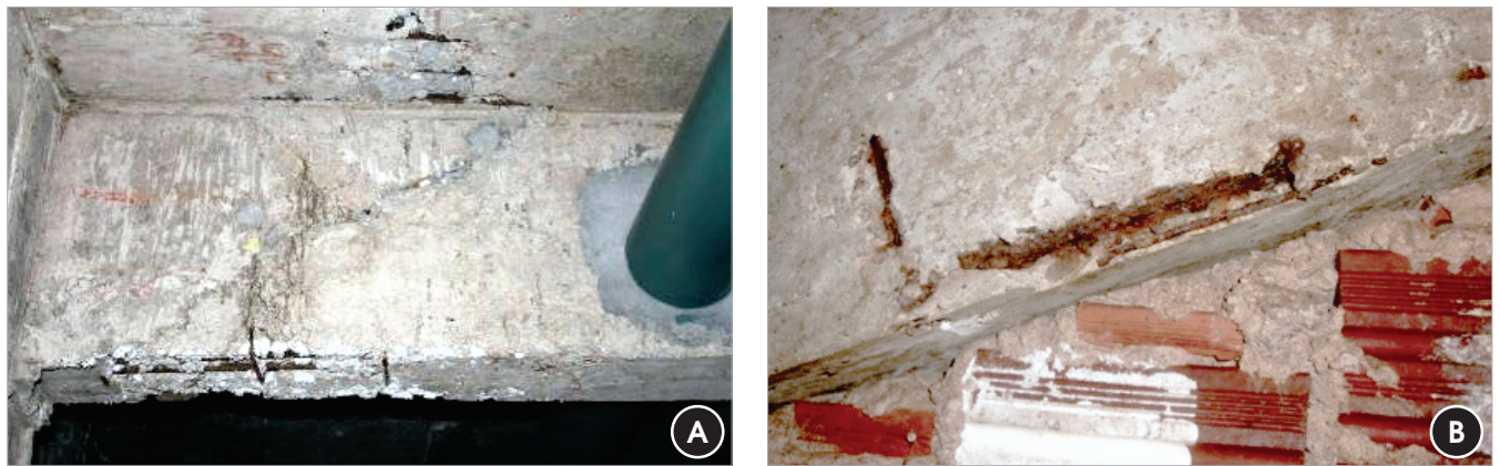
Figure 1 - Aspect of a tensile bottom chord of beam damaged by concreting deficiency and by reinforcement corrosion
