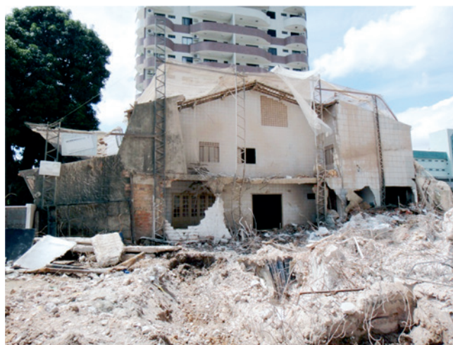
Figure 2 House damaged by the Real Class building debris
