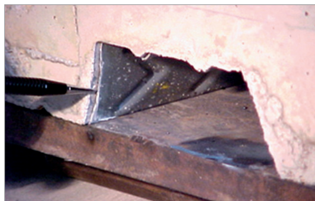
Figure 7 End-slip between the steel sheeting and the concrete
