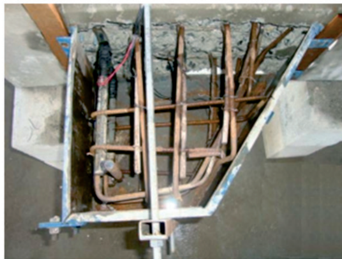
(c) Column-corbelt interface after scarification and reinforcement turned to straight and ready for casting of the corbel (models P3, P4, and P5)
