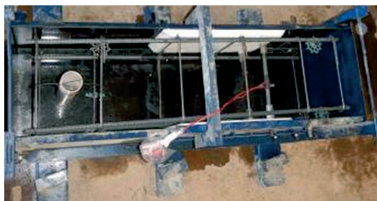
(b) Formwork for casting of column of model with corbel cast in different stage
