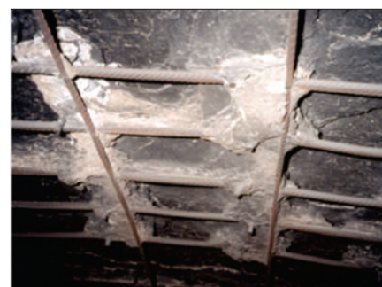
(c) Explosive spalling
