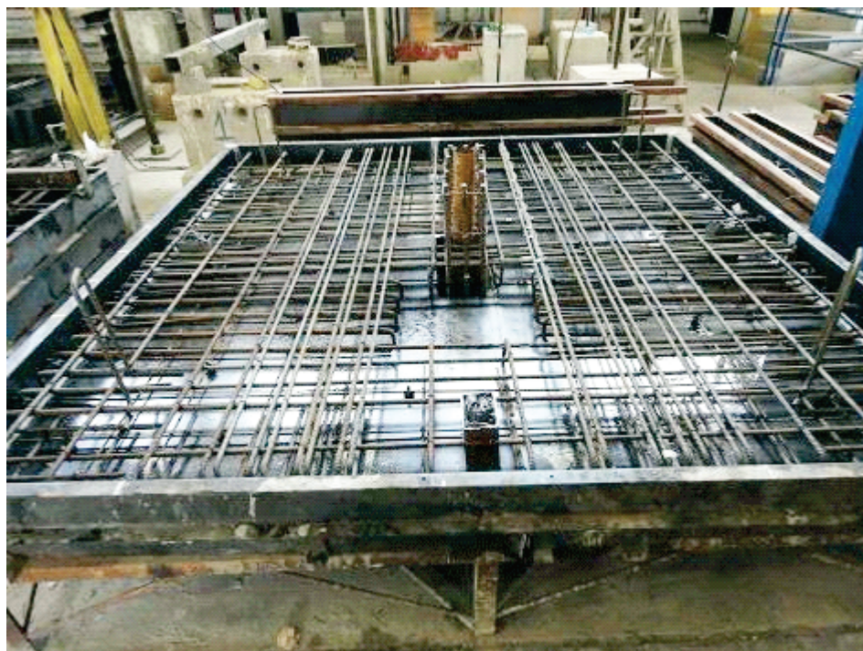
Figure 10 – Photographs of reinforcement placed in metallic formwork (L7 Slab) and moulded-shaped slabs L1 and L2
