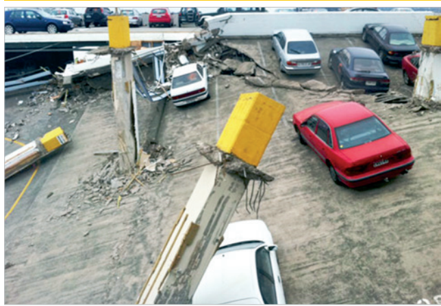
Figure 1 - Punching shear failure of a flat slab floor (Middleton (1))
