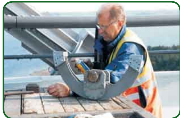
Fig. 15 – Control of the damper components
