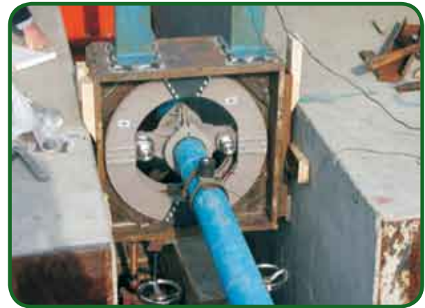
Fig. 12 – View of the VSL friction damper installed on the cable.
