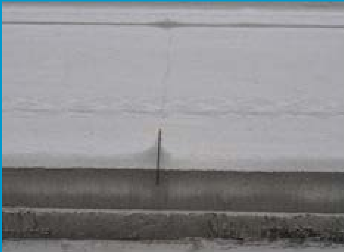
crack at notch
