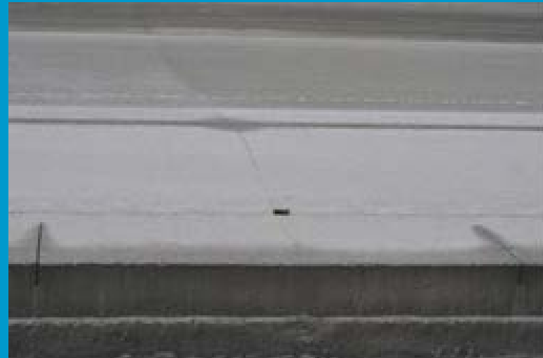
crack in between 2 notches
