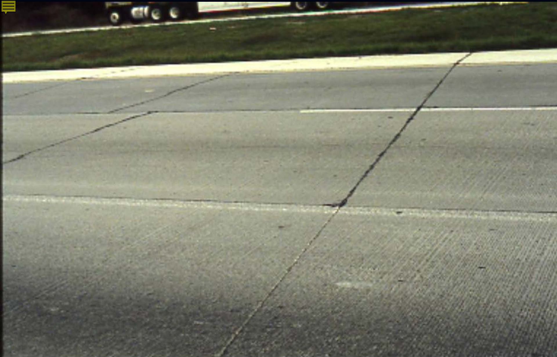
Transverse cracking on I-75 concrete pavement in Florida
